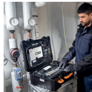
Automatic tightness test
